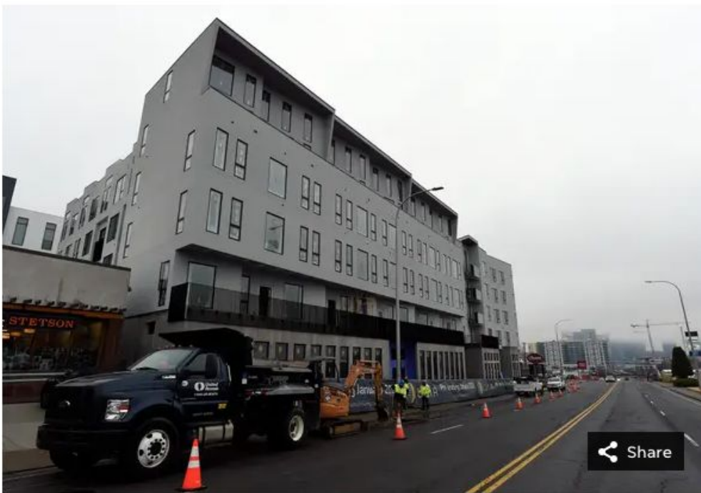
Luna a multi-family development under construction on Monday, Dec. 5, 2022, in Nashville, Tenn. The apartment building is being constructed by Jared Bradley, who is president and founding partner of the Bradley Group, an architecture, development and construction firm in Nashville. MARK ZALESKI / THE TENNESSEAN
